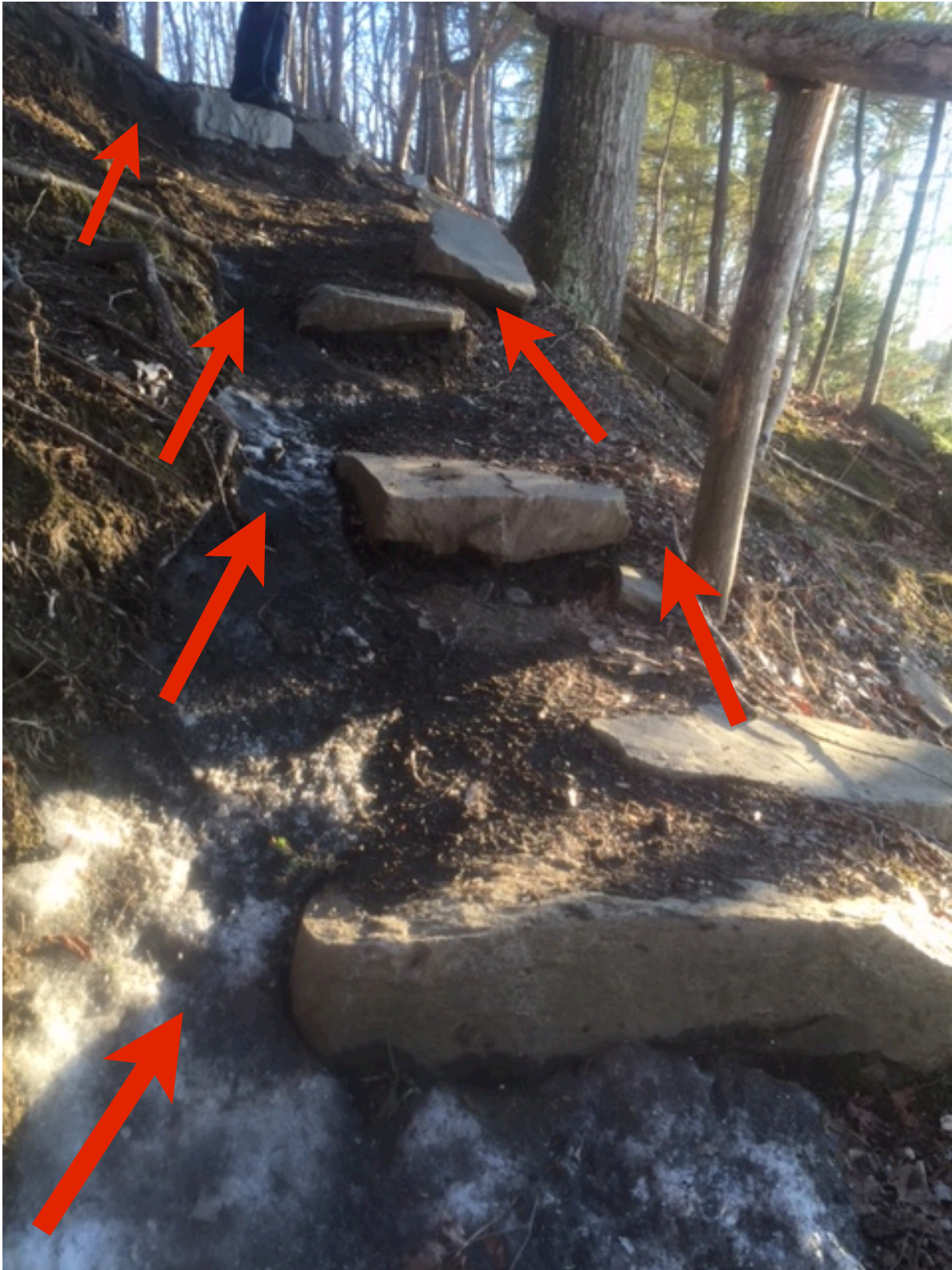
Photo #1: Erosion Around Existing Steps due to Absence of Gargoyle and Crib Stones
